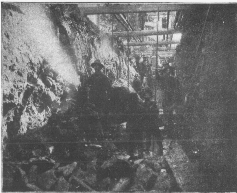
Three out of the ten of our "Ingersoll" steam drills used by Messrs. Laurin and Leitch in excavating rock at St. Louis de Mile End, Quebec. These rock drills are fully described in catalogue No. 81.
