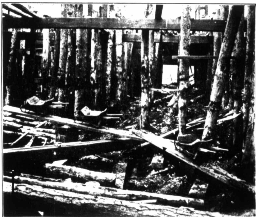
Shewing feet of piles, driven from temporary bracing, before excavation had been completed to point of cut off.
