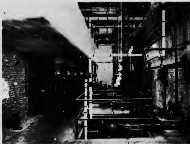
FIG. 10. PUMP ROOM, SHOWING ALSO SMOKE BREACHING IN UPPER LEFT HAND CORNER AND FAN CASINGS IN BACKGROUND. HOT WELL IS IN IMMEDIATE FOREGROUND.
