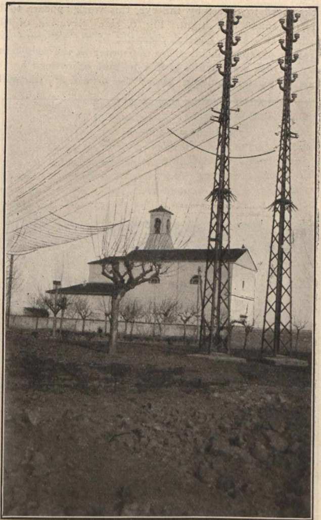
Fig. 4.—Paderno: Transmission Line, showing a Roadway Crossing.
