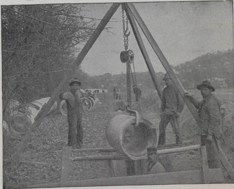
A Triples Block hung from a temporary rigging and used for laying pipe.
