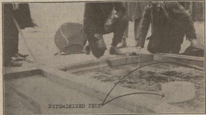
SPACER IN PLACE BETWEEN ROWS OF BLOCK—ROLL OF SPACER MATERIAL IN BACKGROUND
