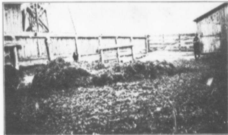
Cut No. 81. Saucer-shaped bottom to barnyard of concrete, preventing loss of valuable liquid manure.
