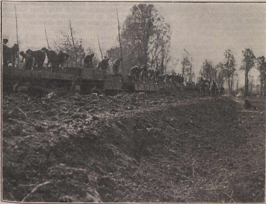
Rapid Railway Construction in France. Building an Embankment for a Broad Gauge Railway. British Official Photograph taken on the British Western Front. Copyright reserved.
