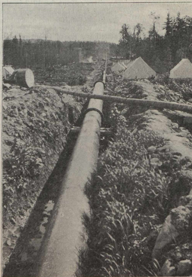
Compressed air pipe line, Gillies Limit, Cobalt
