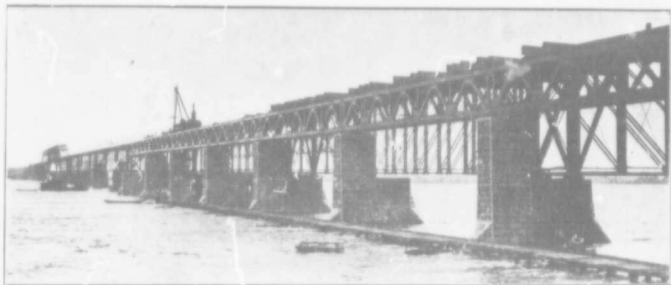
View of the C.P.R. LACHINE BRIDGE showing the work of its double-tracking actually being completed.
