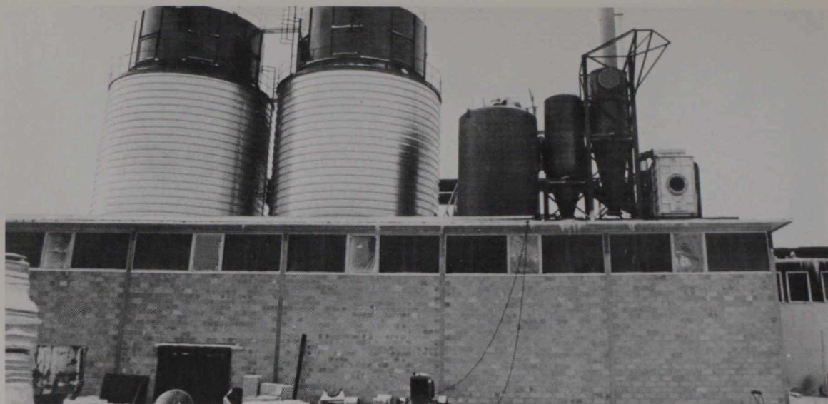
Fluidized-bed gasification converts wood waste to inflammable gas.
