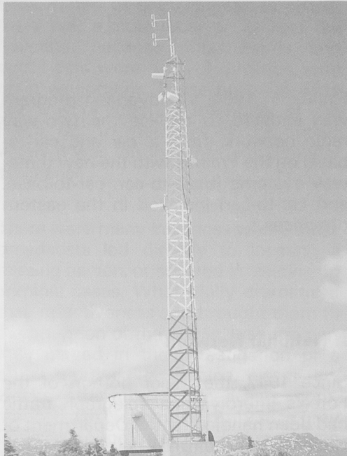
RCMP radio-repeater site with communications shelter and antenna tower at Copper Mountain, near Terrace, British Columbia.
