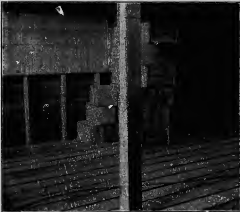
Fig. 7. Basement of Dr. Whitney's Wenatchee Valley storage, showing floor and wall construction.
