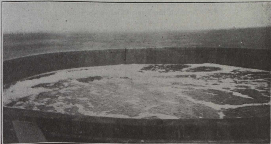
View of Top of Activated Sludge Tank in Operation, Showing the Even Character of the Air Distribution.
