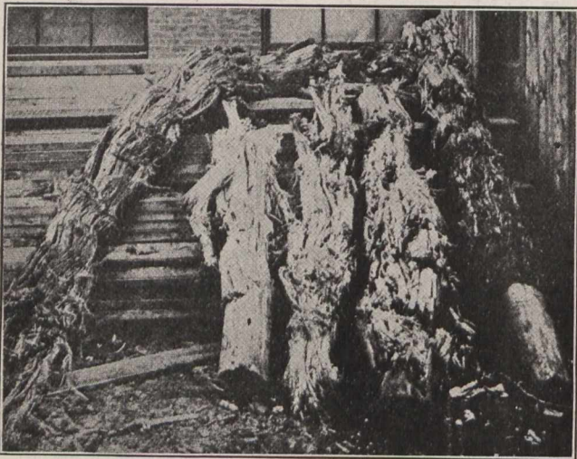
Fig. 1.—“Broomed” Wooden Piles, Supposed to be in Good Condition, Until Excavated for Inspection.
