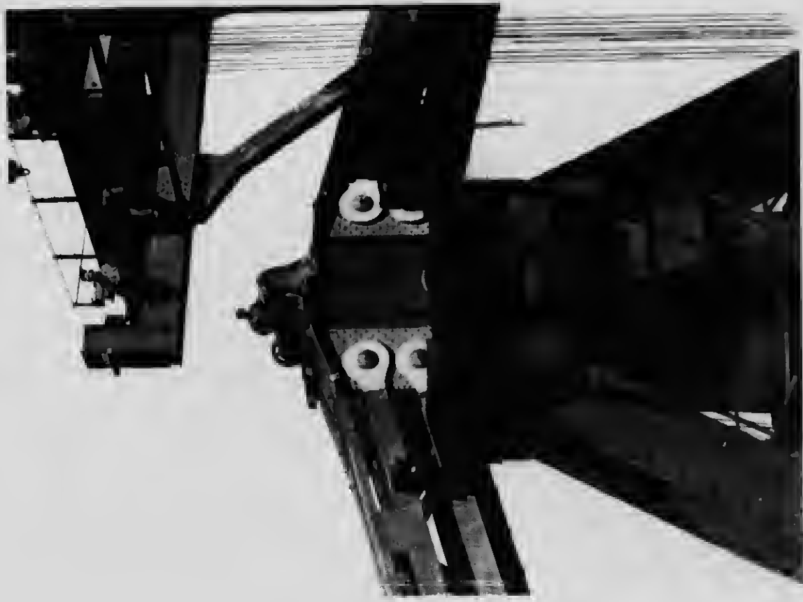
55 Detail of the large link and connection at the top of the main pier post
