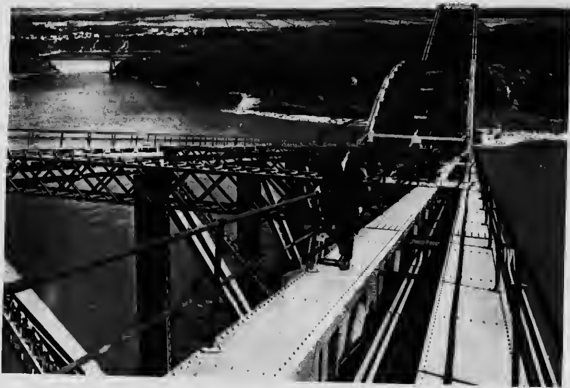
76 View from the top of the N W Main Post, showing inspector's walk, which is reached by means of 12 steel stairways
