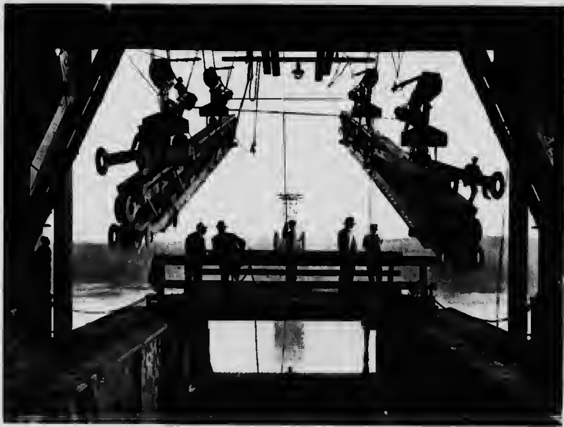
38. Another view of the upper chord eyebars being hoisted, assembled in the supporting box girders. Shows in the distance the South Shore traveller erecting the lower triangles of the South Shore anchor arm truss
