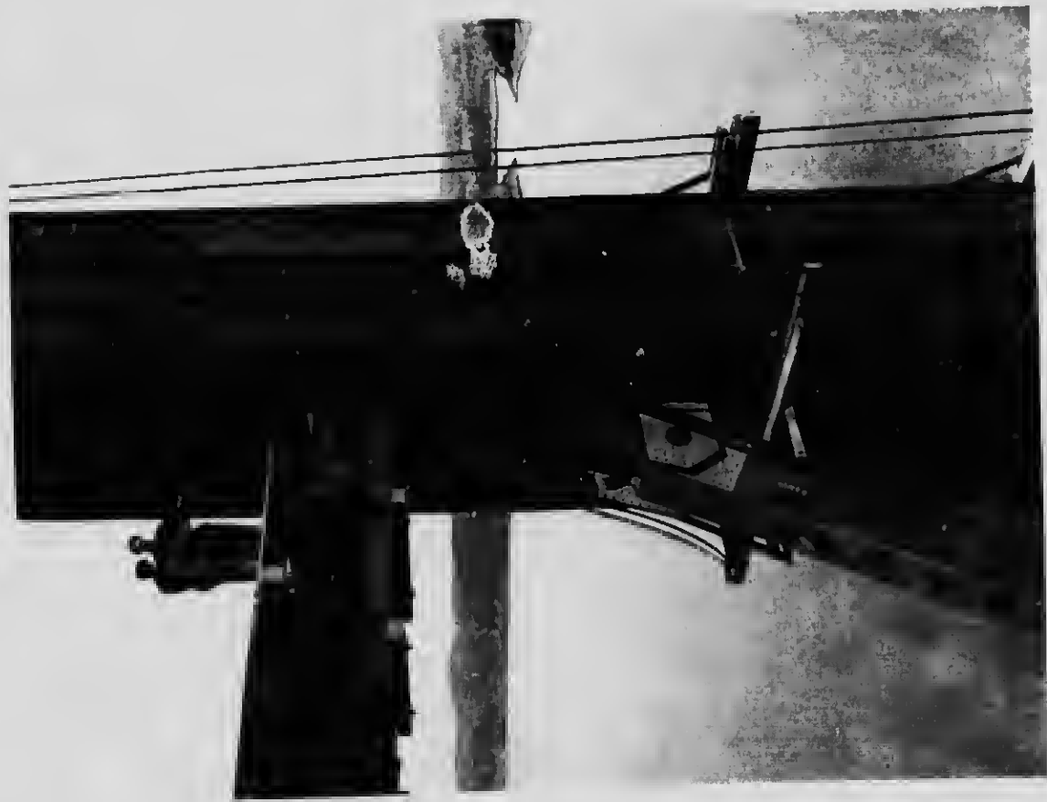
27 Connection of web members at the centre of the large pier over the main pier
