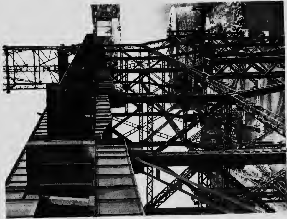
18. Permanent track girders and flow beams supported by the falsework; also shows the hatched pin holes in the end of flow beams.
