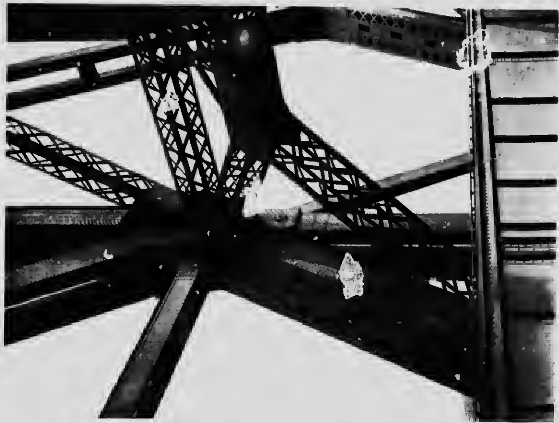
74 Detail at 6.5M 14 The middle panel point of the cantilever Arm adjacent to the Main Post
