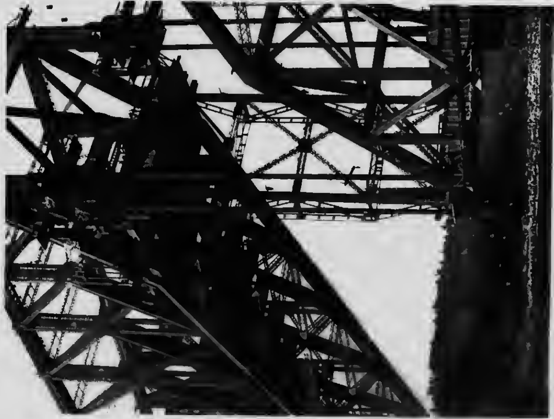
54 General view of the bolting and moving apparatus; also shows permanent eschar hangers in place, the lower half of them on the suspended span and the upper half suspended from the outer end of the cantilever arm.
