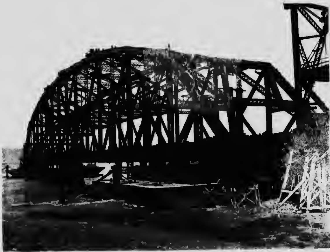
58 The suspended span resting on the end supports at Silery. The falsework removed and the scows bucked under ready for floating.
