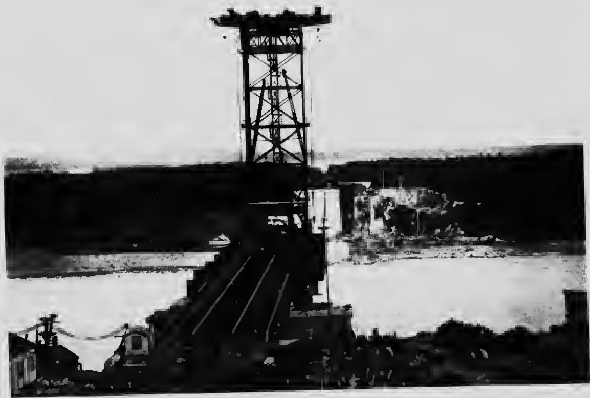
17 End elevation of the traveller at the same position as on plate 16, showing the four tracks on which it was carried and the temporary outside girders to support the outside tracks
