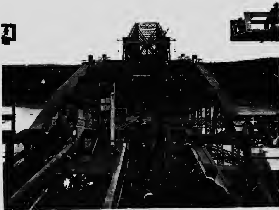
67 The top of the suspended span appearing above the cantilever floor, September 18th, 1917
