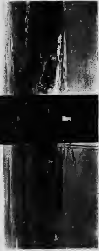
28 Placing one section of the large link at the top of the main pier post
