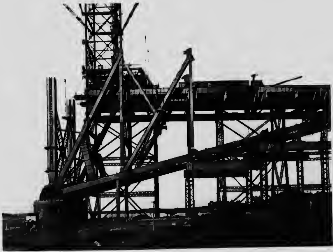
24 Two lower triangles of the web system of the anchor arm erected
