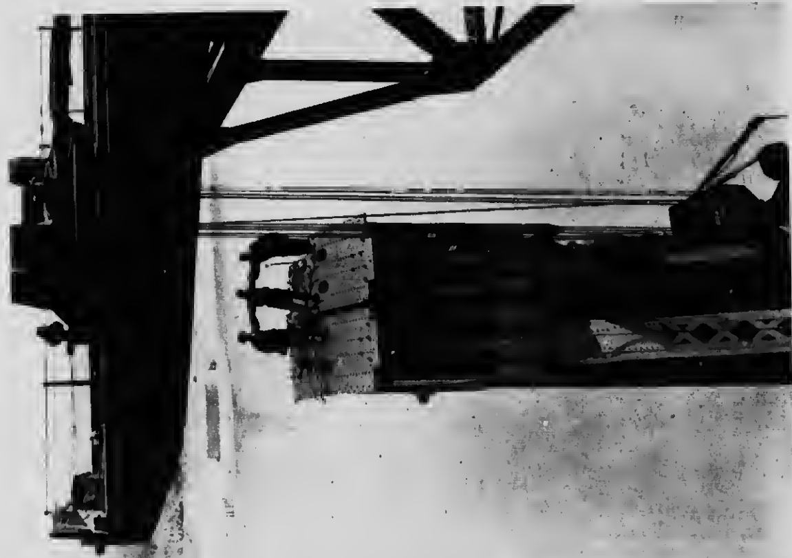
20—The large link at the top of the main pier post is placed
