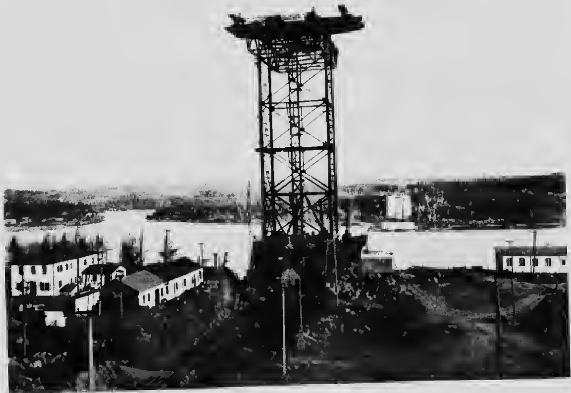
15. The North Shore traveller erected being equipped, also showing the office building and power house to the left
