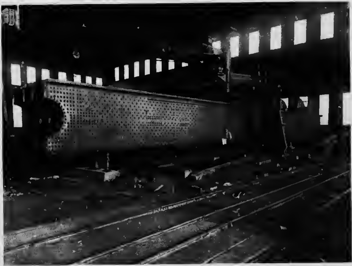
12 Pier panel of the bottom chord assembled for drilling the splice connection holes
