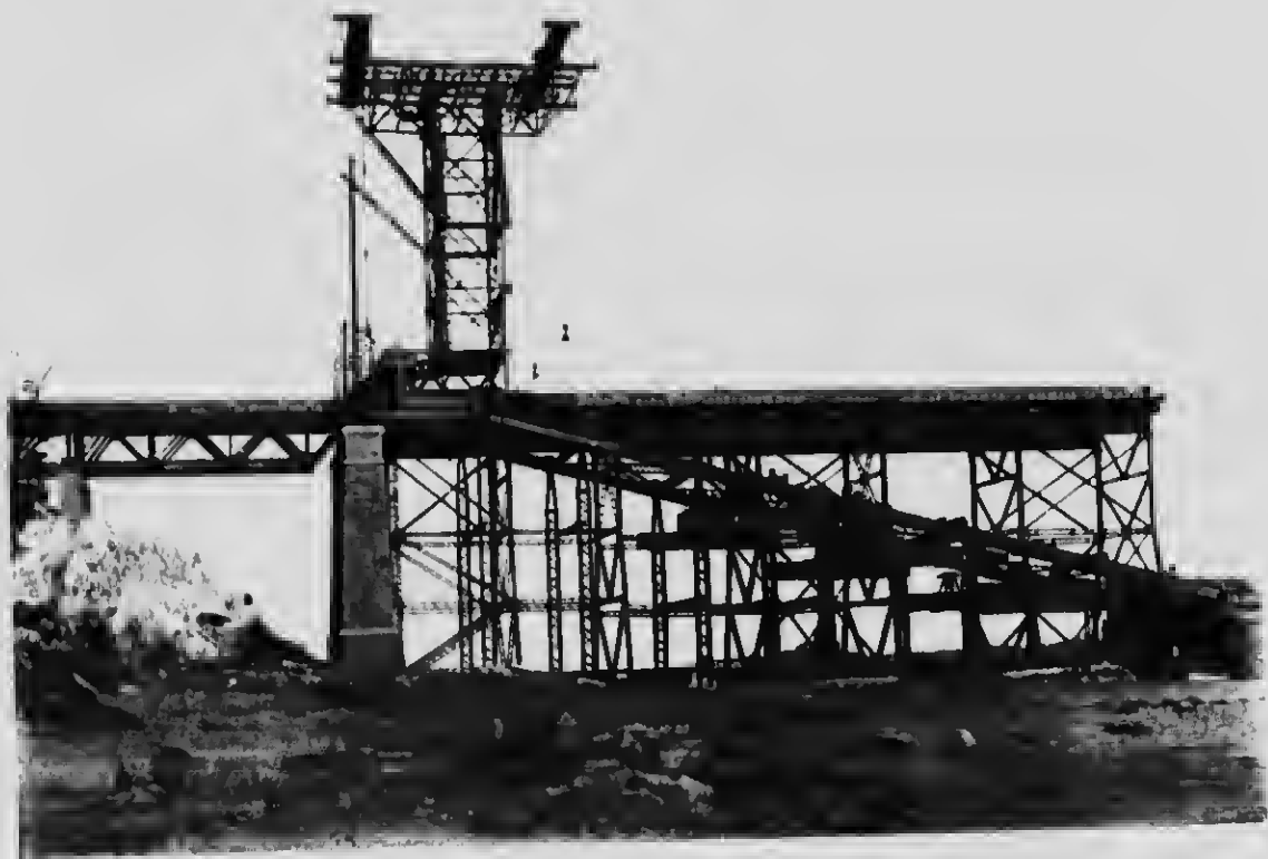
22 The anchor arm lower chord completed. Lowering anchor bars into the wells of the anchor pier
