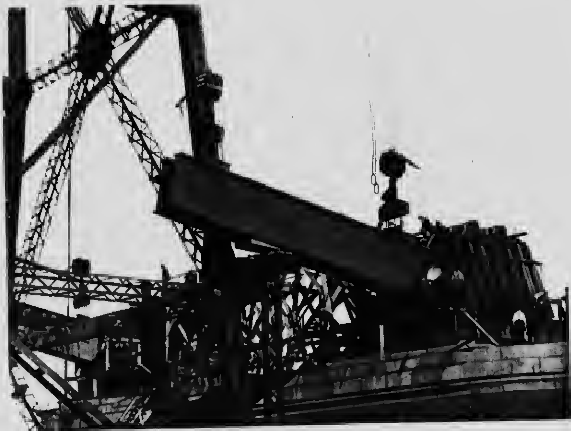
26 The Northwest shore is erected complete except the cover plates over the stiffening ribs. The first section of the lower chord of the anchor arm is being placed
