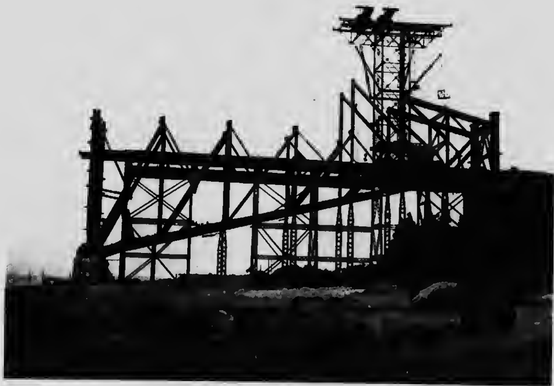
25—All of the lower triangles of the anchor arm erected. Starting the erection of the upper triangles and upper chord
