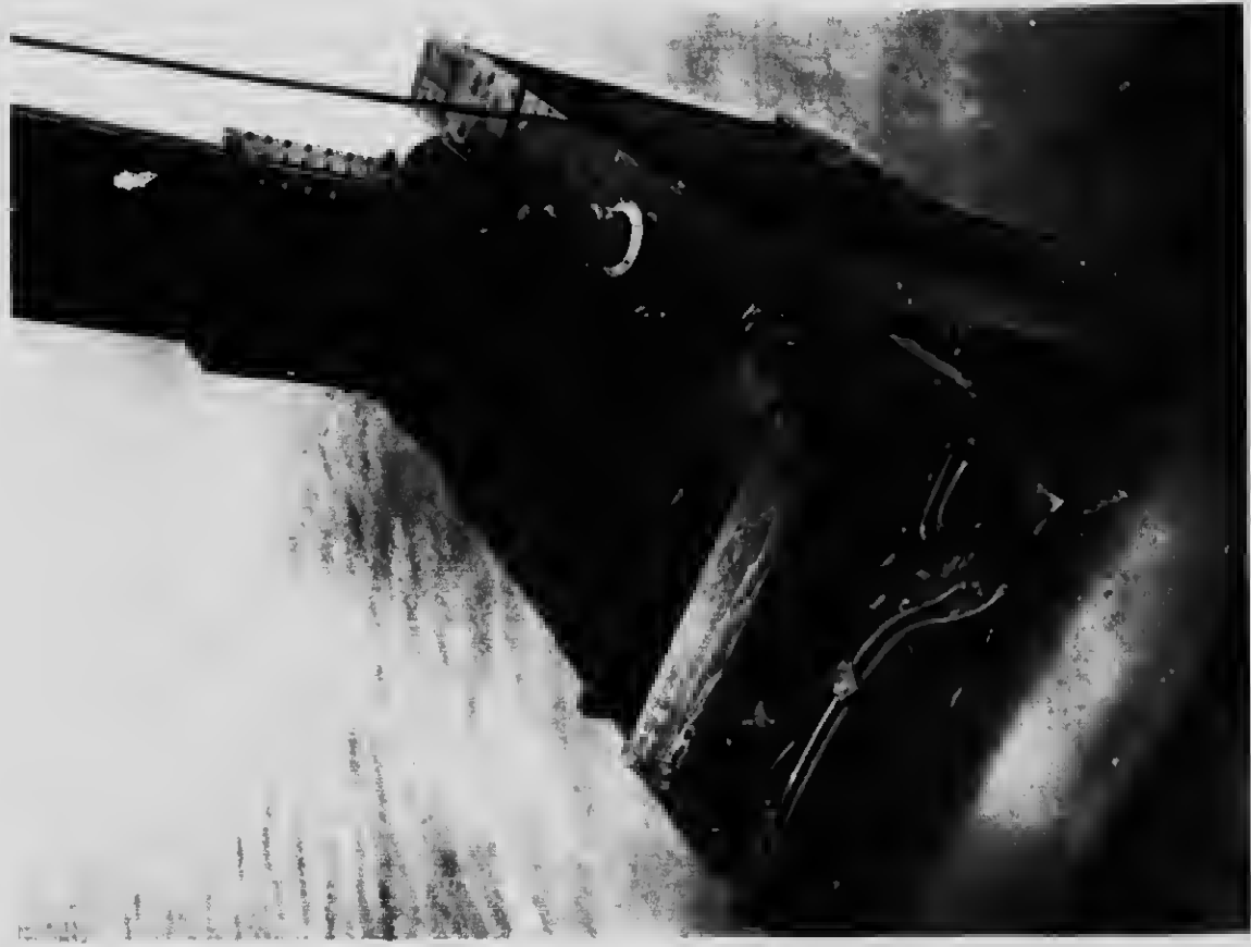
65 Condition of lower show and carrying glider after the loss of the suspended span
