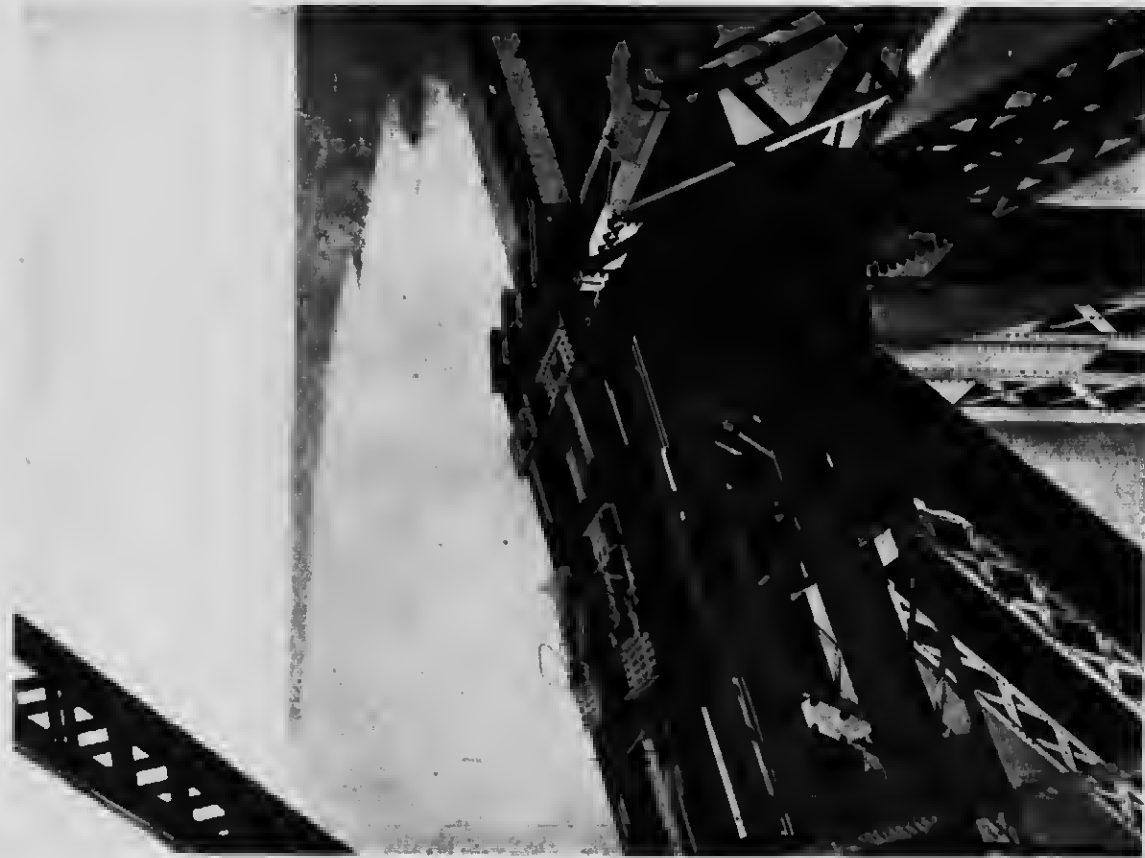
40 Detail of the temporary connection for holding the upper chord eyebar supporting girders in place and for adjusting the pin hole centres.
