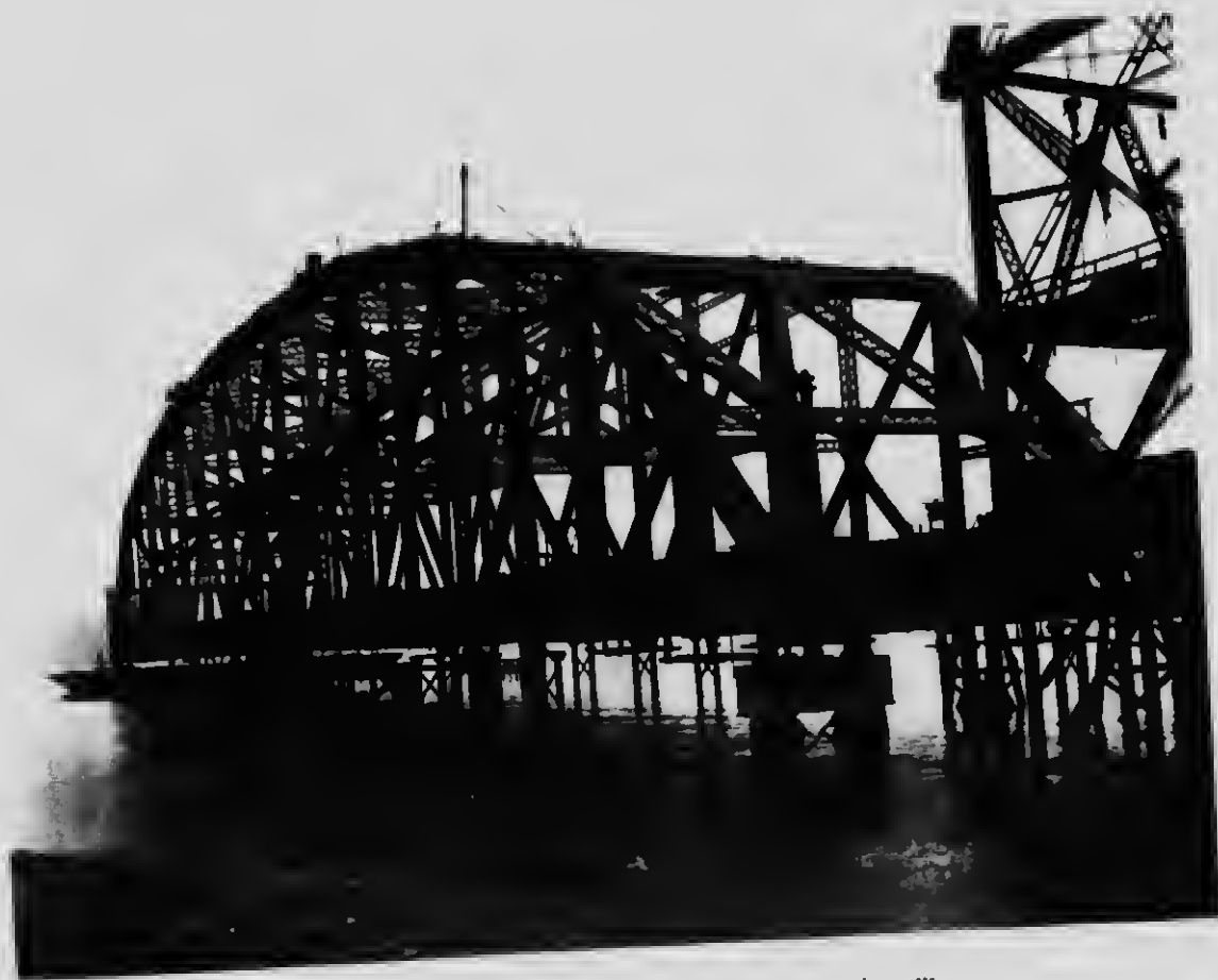
49 - The falsework removed with the suspended span resting on the end supports
