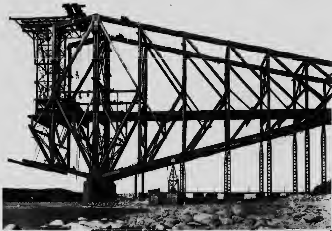
14 The first half of the second panel of the cantilever arm erected
