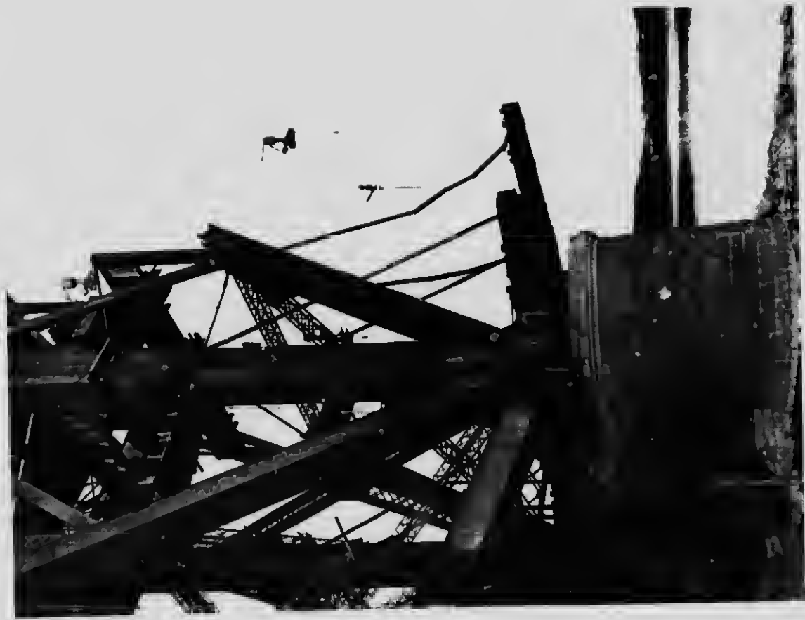
31 -Starting the erection of the North Shore cantilever arm, showing the supporting platform in place carrying the first sections of the lower chord
