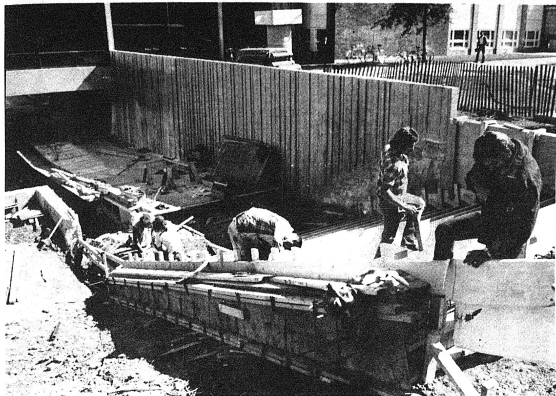
Work delayed on ramps...
