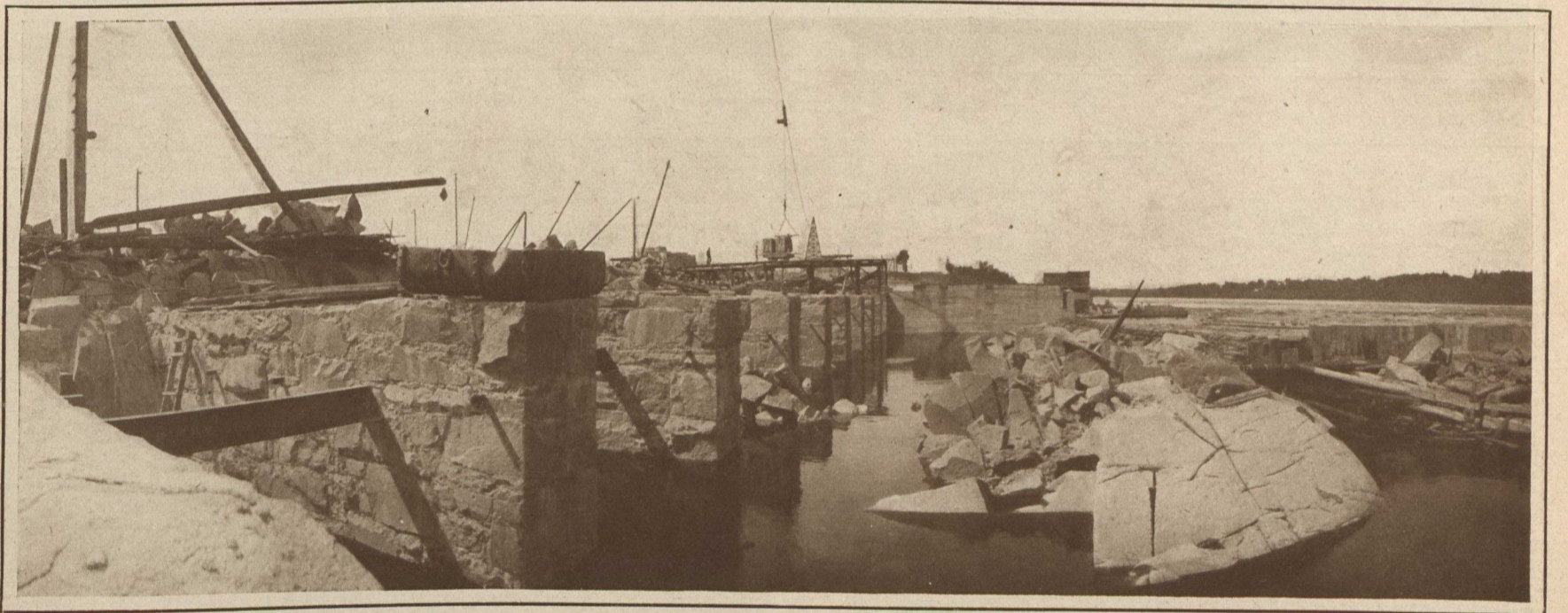
A Modern Dam is Wonderful as Compared with those Built in Canada in the Early Days of Last Century.
