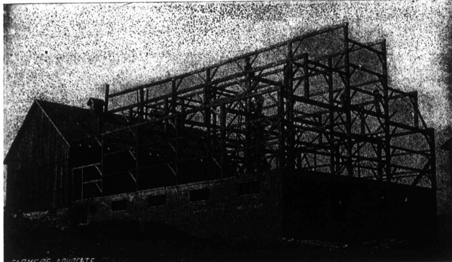
Basement and Frame of Mr. J. A. James' Dairy Stock Barn, Nilestown, Ont. New portion, 72x60 feet. Walls, 12 feet high.
