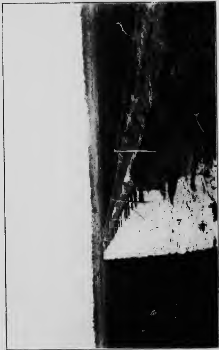
Showing clean cut of a working trench made by the Anrep excavator at Alfred, Ontario. (Note the even slope).
