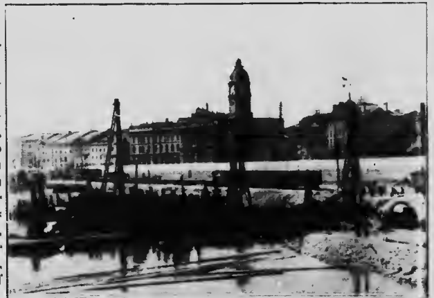
The Transformation of Montreal Harbor. The Piling for the Harbor Commissioners' Elevator, June, 1902.
