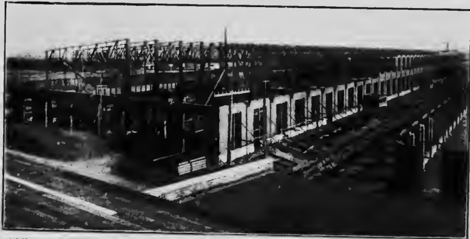
Lessard & Harris, Builders. Machine and Erecting Shop in process of erection at the New C. P. R. Shops, Montreal. The Largest Building under One Roof in Canada.
