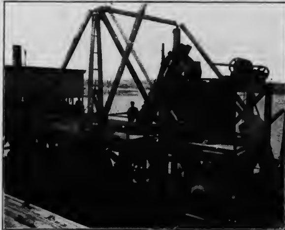
Partial View of Floating Concrete Plant, Equipped with No. 3 Smith Concrete Mixer and No. 6 Austin Gyrotory Crusher; showing Front View of Mixer and Top of Crusher in Centre of Platform
