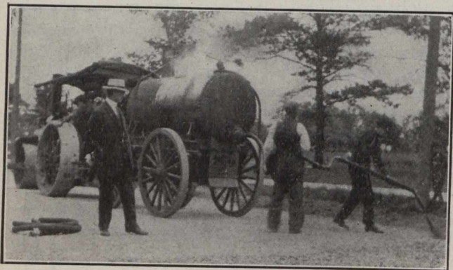
Fig. 4.—Tarvia "X" Being Distributed from a Tank Wagon Fitted with a Fire Box and Hose Attachment.
