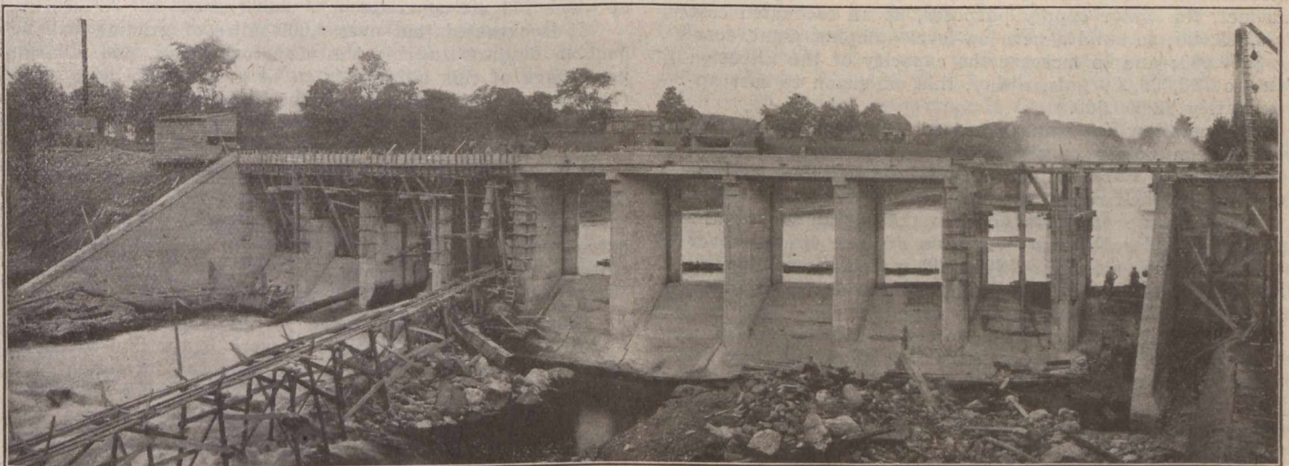
FIG. 7—DAM UNDER CONSTRUCTION—PART OF MIXING PLANT AT EXTREME LEFT—TRESTLE TO POWER HOUSE IN LEFT FOREGROUND
