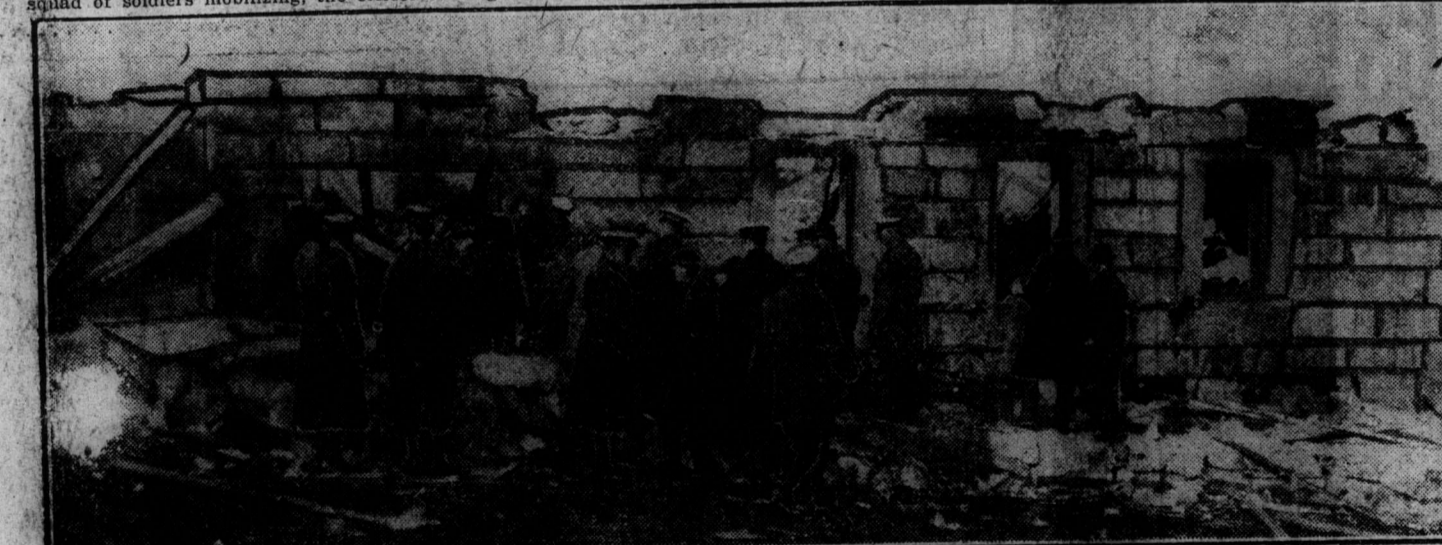
ANOTHER VIEW OF RICHMOND PRINTING CO.'S BUILDING. This plant was situated on Old Campbell road and when it collapsed 30 girls and several men lost their lives. A wrecking party including a number of soldiers, are already beginning the seemingly hopeless task of shifting some of the debris in an effort to find the bodies.
