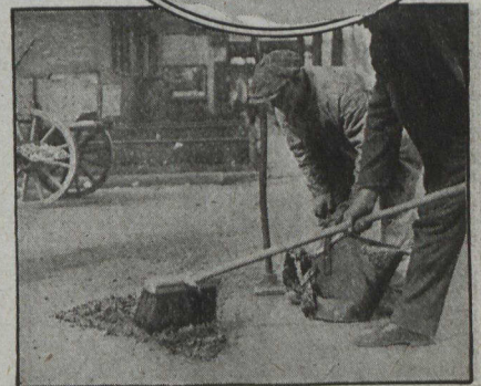
A seal-coat of 1/2 gallon of "Tarvia-KP" to the square yard is spread over the patch.
