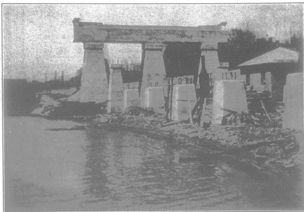
Concrete piers recently completed for bridge over railroad at Sunnyside, Toronto, Ont. Crushed stone and cement supplied by Alfred Rogers, Limited.
