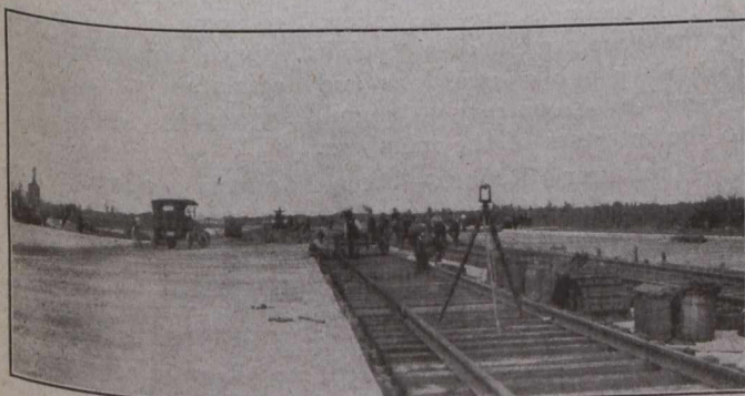
Fig. 5.—With Track to Grade, Filler is Poured up to Bottom of Proposed Pavement.
