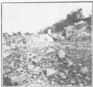
Deviation used in Valsch River during the War, when Kroonstad Bridge was destroyed.
