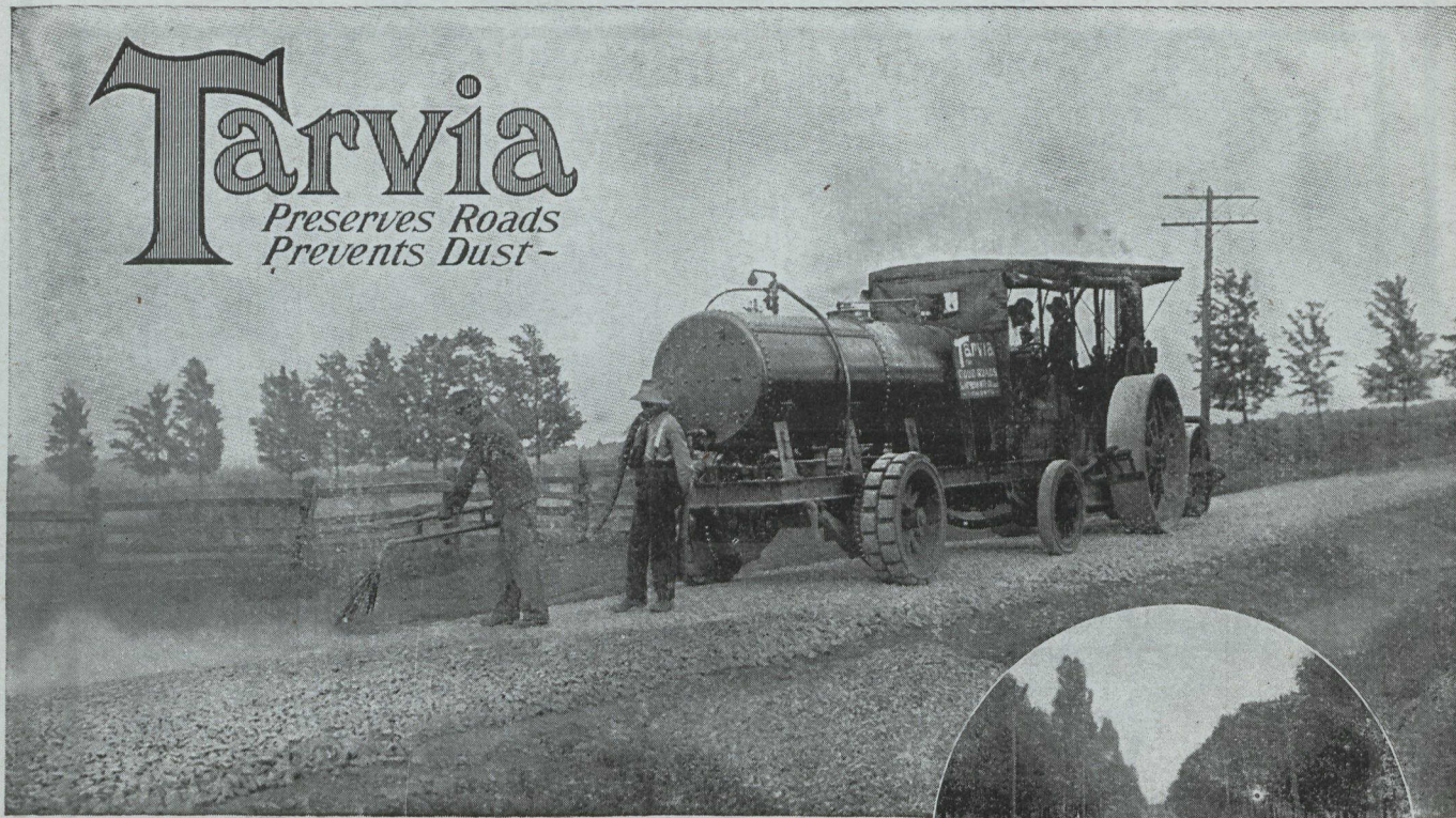
The above illustration shows the spraying of hot "Tarvia-X." The view in the circle is the finished road. It is durable and dustless.
