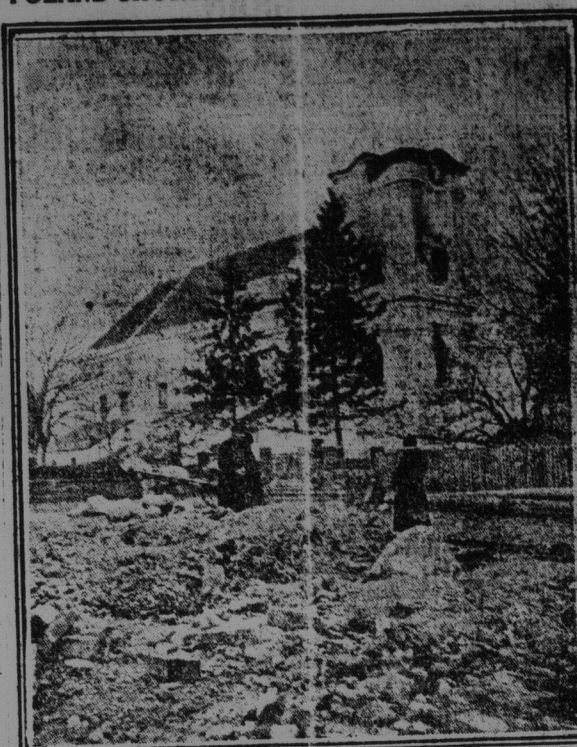
DAMAGED CHURCH OF MAKOV, POLAND. This little Poland town has suffered from shell fire during the collisions of the Russian and German forces.
