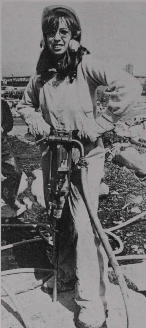
Danielle Trush uses a jackhammer to break up rocks. The girls were among a dozen young women working on Vancouver's False Creek breakwater project, the first women labourers the city has ever hired.
