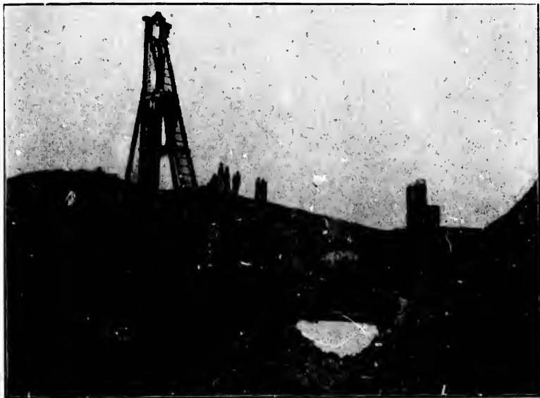
The Pile Driver at Work on Construction of Headgates at Intake of Irrigation Canal.
