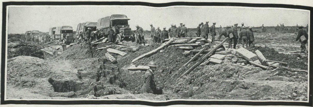
When the Canadians cannot wait for light railways they build cordwood roads. This is the improvised road on which they followed up victory across Vimy Ridge
