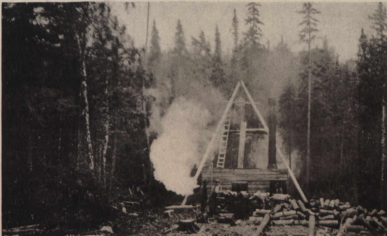
Recent Photographs Showing Mining Developments in the Wasapika Gold Area of Northern Ontario. A Newly Opened and Promising Goldfield.
