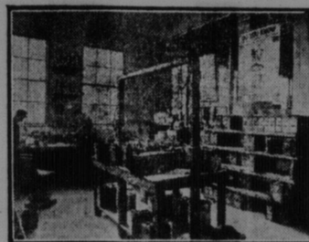
A VIEW OF BATTERY ROOM.
