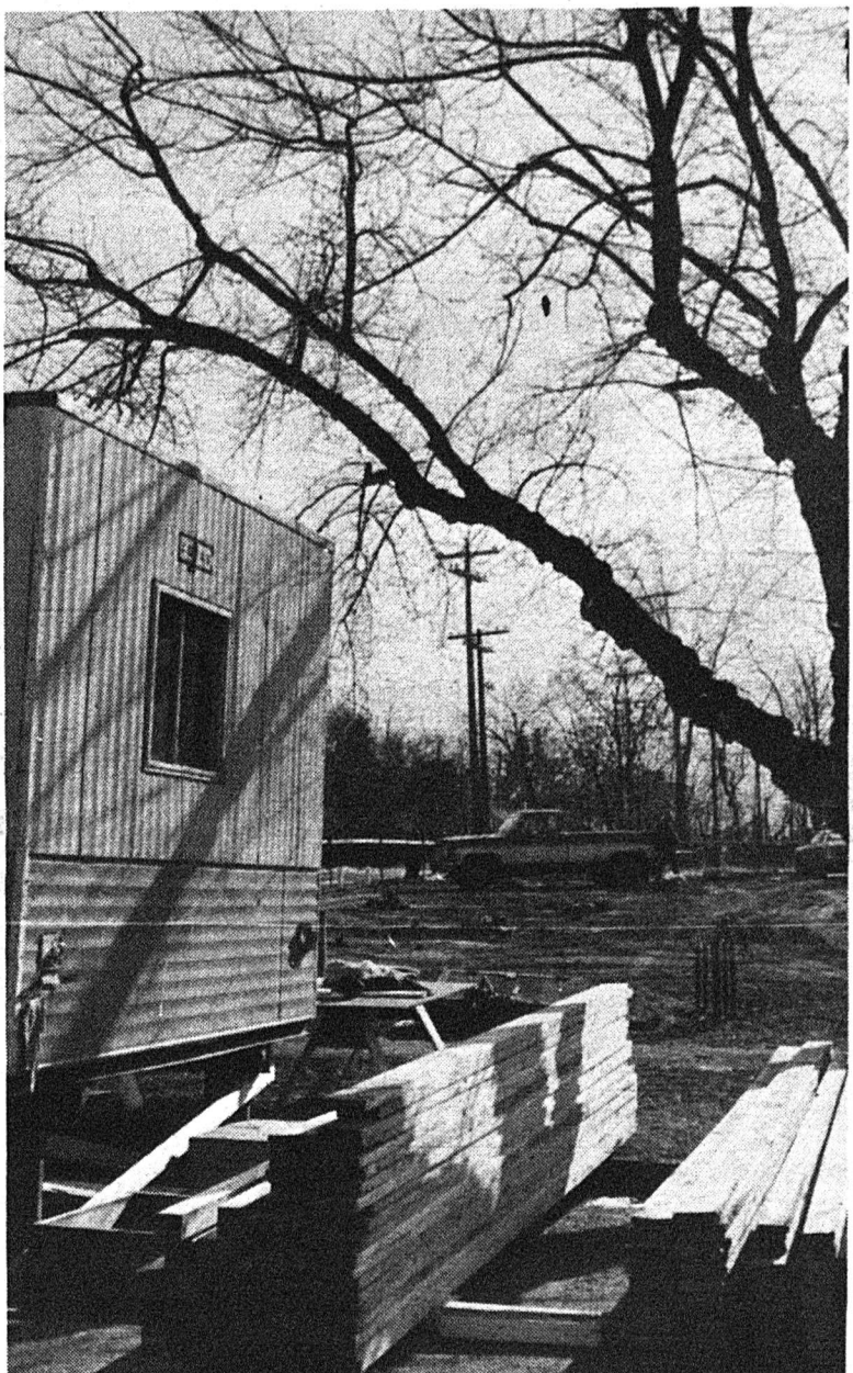
A temporary structure to house university health services (which has been displaced by construction at the University Hospital) is being erected in the parking lot directly south of the Law building, on 111 St., between 87 and 88 Avenue. photo by Shirley Glew
