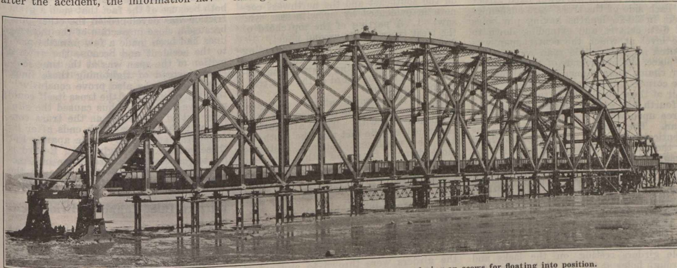
Quebec Bridge—Suspended span erected on shore at Sillery Cove, prior to placing on scows for floating into position.
