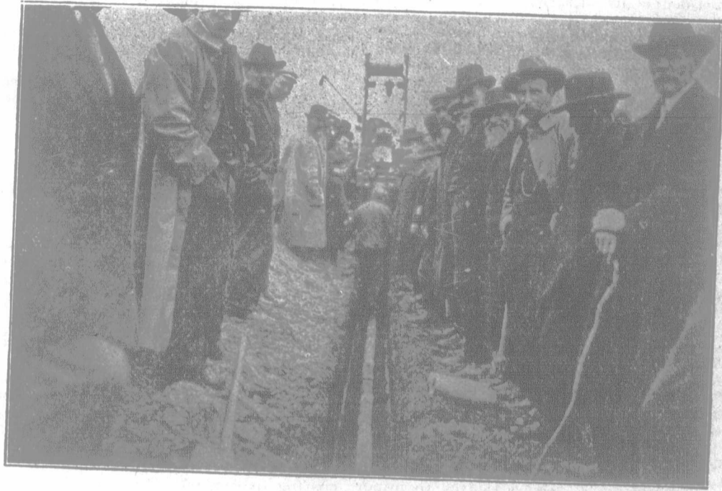
Crowd Watching the Ditcher Work. Drainage demonstration on the farm of Neil McDougald, Tara, Ont.
