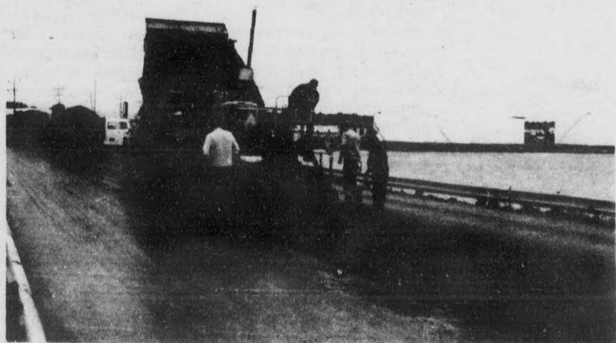
Ice Free pavement courtesy The civil department
