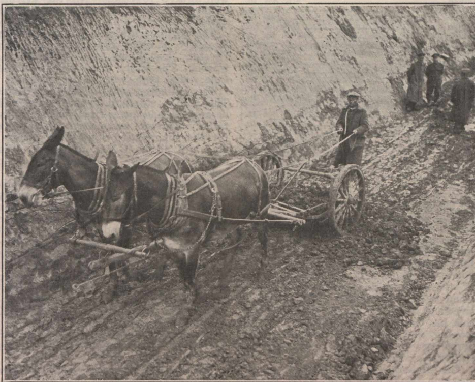
Canadian light railway construction on the British Western Front. The scraper filled, on its way to end of embankment. Canadian Official Photograph. Copyright reserved.
