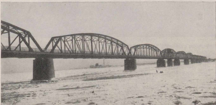
Fig. 13 represents the railway bridge over the Yalu River between Manchuria and Korea—evidently a pin-connected structure and, therefore, not quite up to the latest American practice April, 1930.
