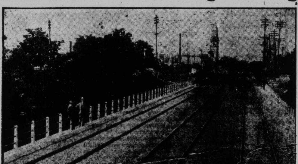
The double tracking of the North Toronto Sub-division of the Canadian Pacific Railway between Leaside and North Toronto is now nearing completion, and involves the replacement of bridges (known as O.S. and L.S.) which heretofore had been trestles constructed of steel.
