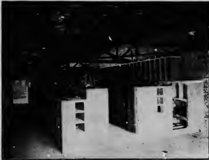
TORONTO TRANSFORMER HOUSE, SHOWING OIL SWITCHES.
