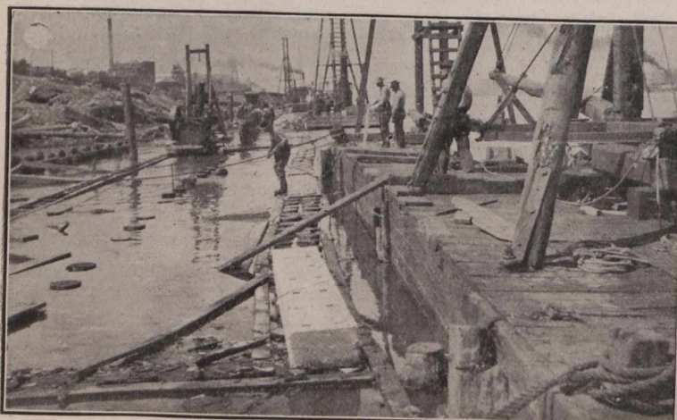
Anchor Piles Sheeted and Rotary Saw at Work on Rear Row of Bearing Piles.
