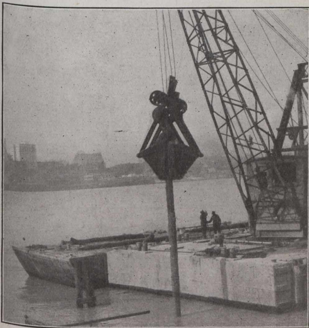
Extracting Old Piling With Dredge at Windsor, Ont. Submerged Cribwork on Site of New Government Wharf Prior to Its Construction.
