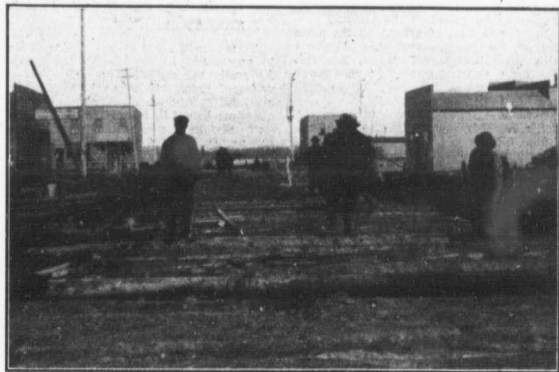
LAYING CORDUROY ROAD, SOUTH PORCUPINE. Amateur photo. Negative by Mrs. W. J. Brown, Shallow Lake, Ont.
