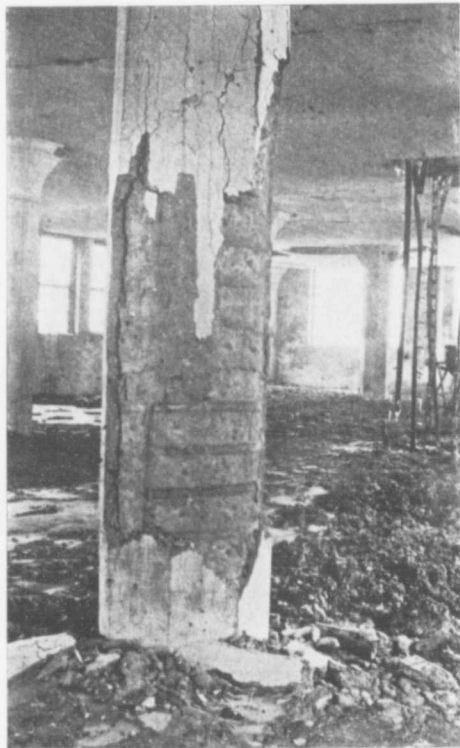
Fig. 3. Spalled column and unprotected bag hoist on right.
