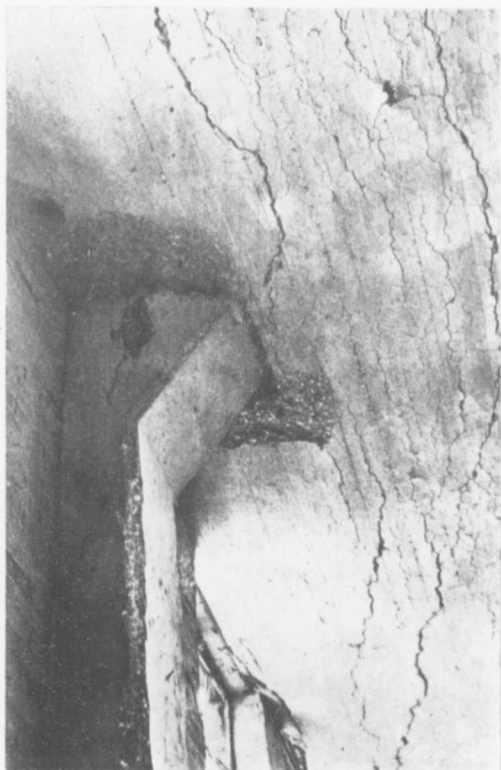
Fig. 13. A column which forced its way through ceiling.
