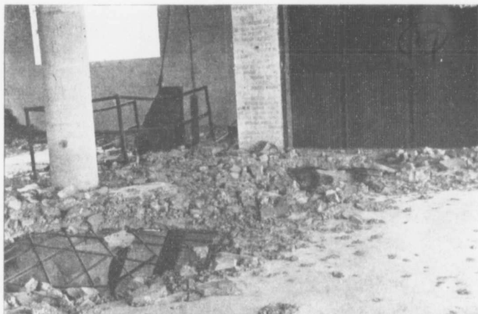
Fig. 16. Corrugated steel doors in elevator shaft. Note also condition of wood tin-clad trap at stair opening on left,
