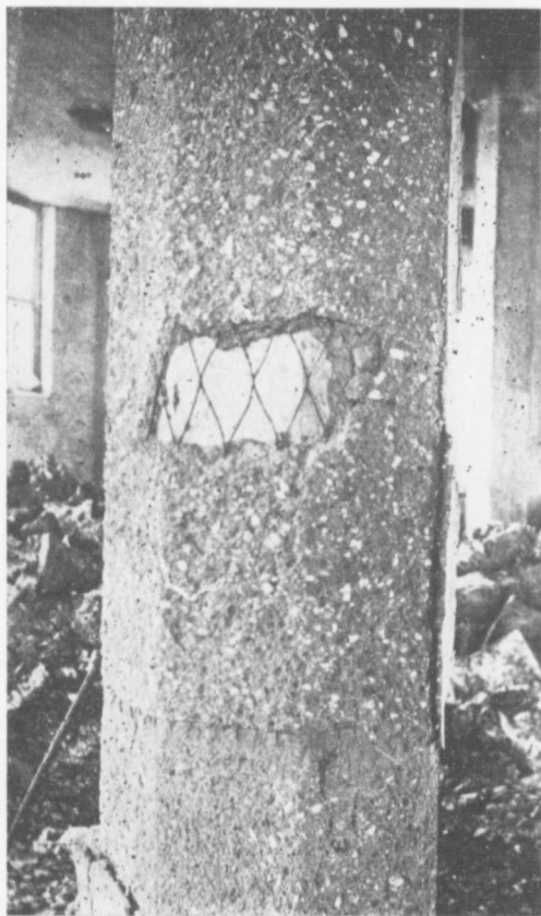
Fig. 11. Column which had been thickened by pouring of additional concrete. (See page 32)
