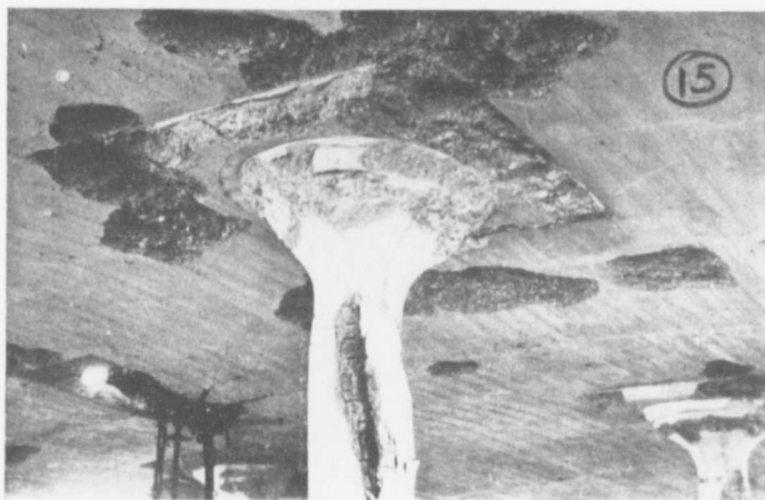
Fig. 12. A column failure.
