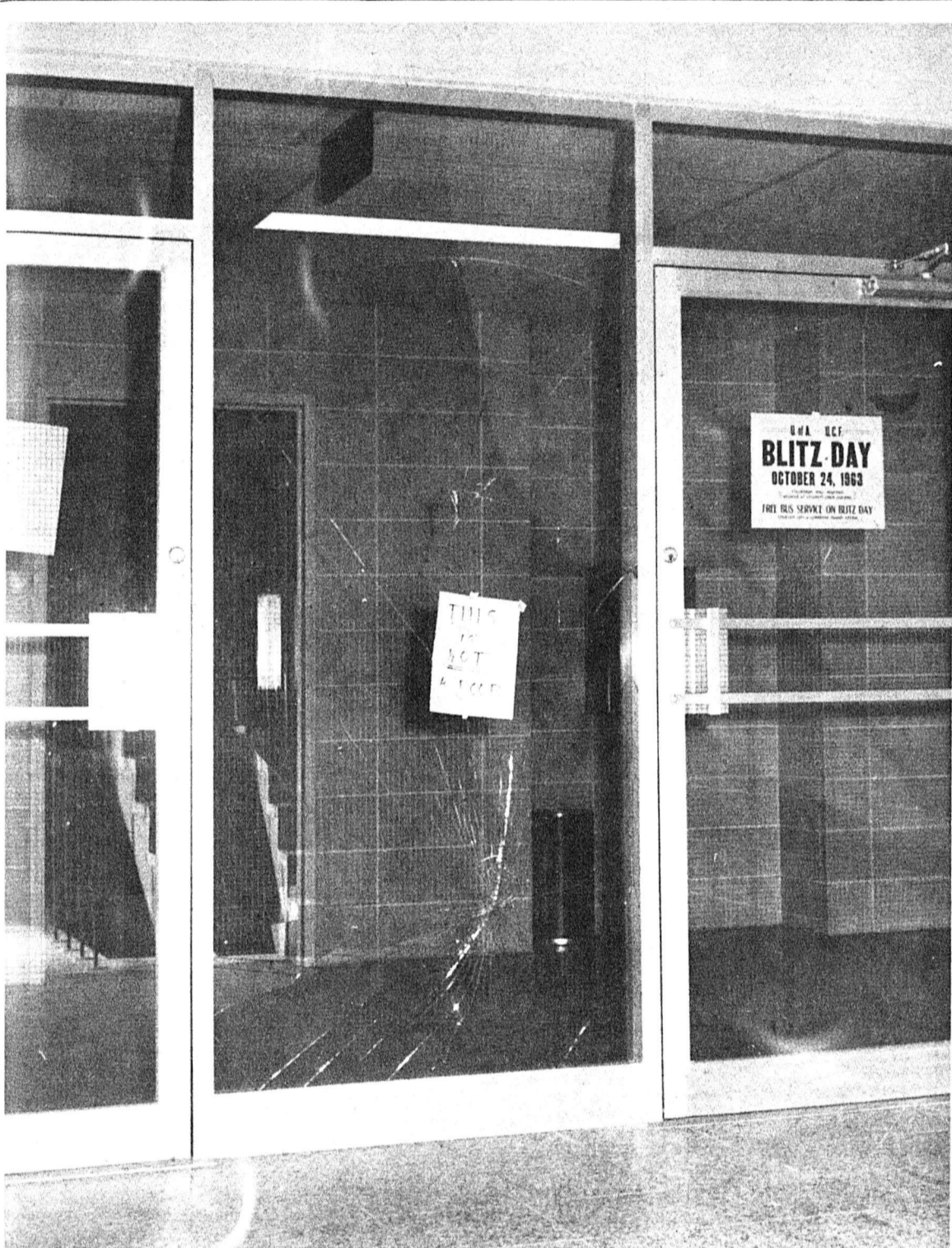
PROGRESSIVE EDUCATION?? —An unheeding unreading Education student knickety splitted thru a panel that was unfortunately there to manifest a spider web in the multi-million dollar building. Broken doors? Stairways to nowhere? Cracks in the walls? A forecast from an uninformed source predicts the Ed Building will fall before Christmas.
