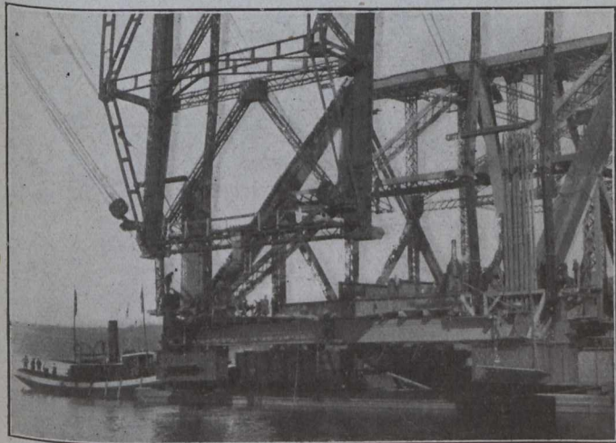
Fig. 1.—Connecting the South End Hanger Chain to Sub Links of Lifting Girder. Engaging the Leafs Before Driving Lifting Pin
