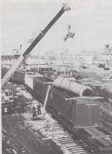
At CN Rail's Pointe St. Charles yard, the length of special slinging gear made yard derrick unusable, so an extendible-boom crane was brought in for the unloading.
