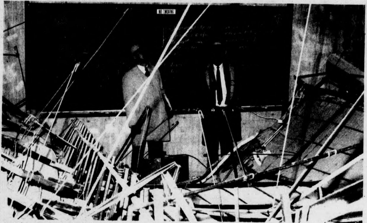
Two fire safety inspectors examine damage to Curtis discussion room 110 after last week's cave in.
